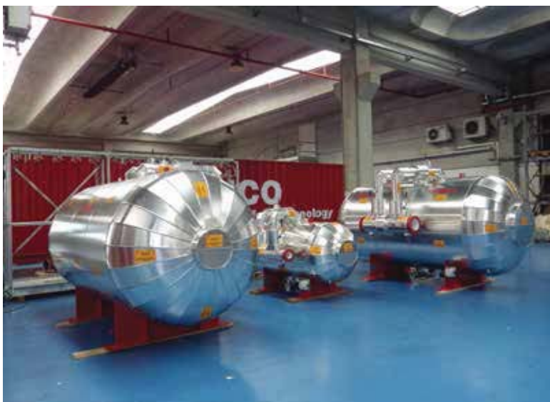
Fig. 5 - Uzbekistan project: foam bladder tanks with thermal insulation for very low temperature
