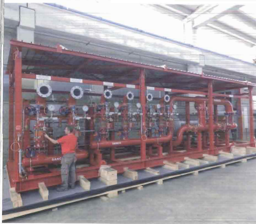
Fig. 2 - Deluge valves on skid
