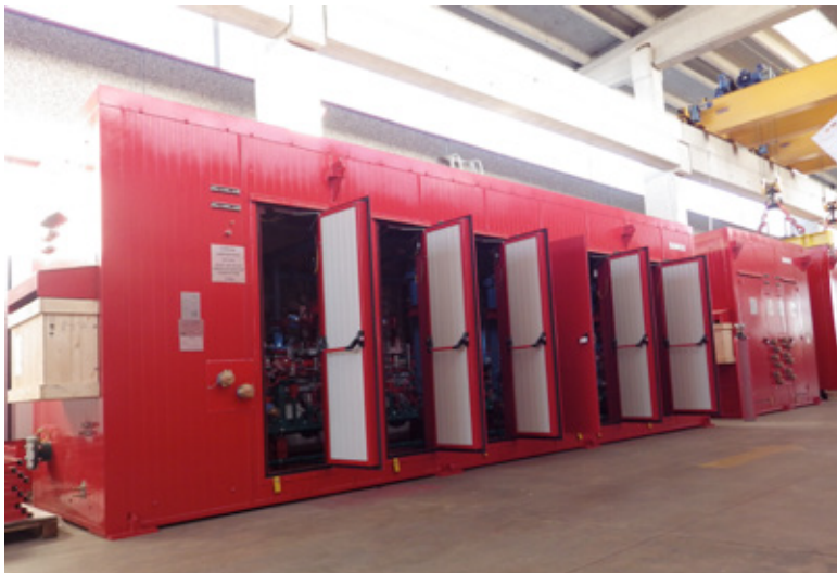
Containers view with opened safety doors
