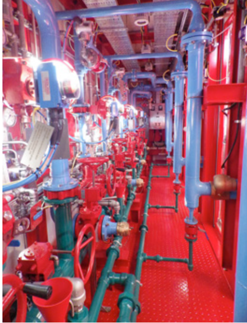
Deluge valve: typical container, interior layout
